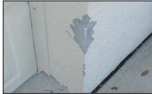
Damage near garage
