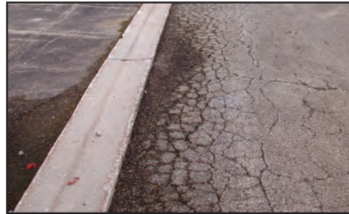
Alligator cracks and settlement at edge of access drive
