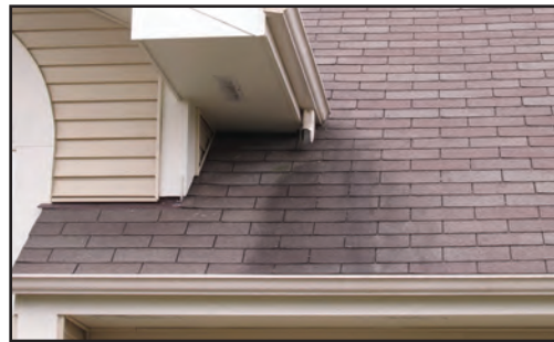
Downspout discharge directly onto shingles
