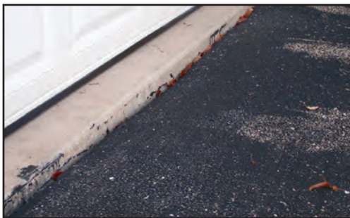
Settlement at garage threshold
