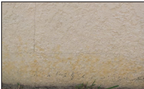
Crack at side elevation
