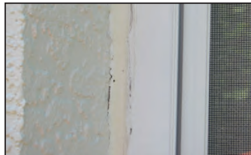
Sealant adhesion failure
