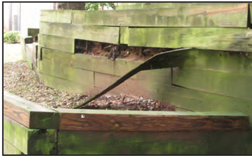
Wood rot and wall deflection
