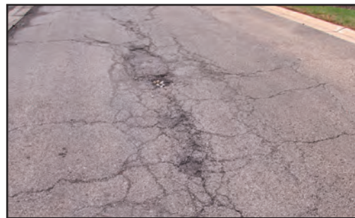
Cracks and potholes
