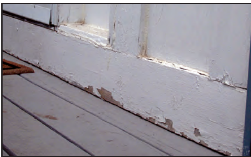
Paint finish deterioration
