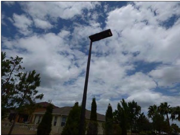
LED Playground Lighting
