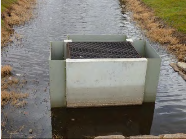
Stormwater Drainage Control Structure
