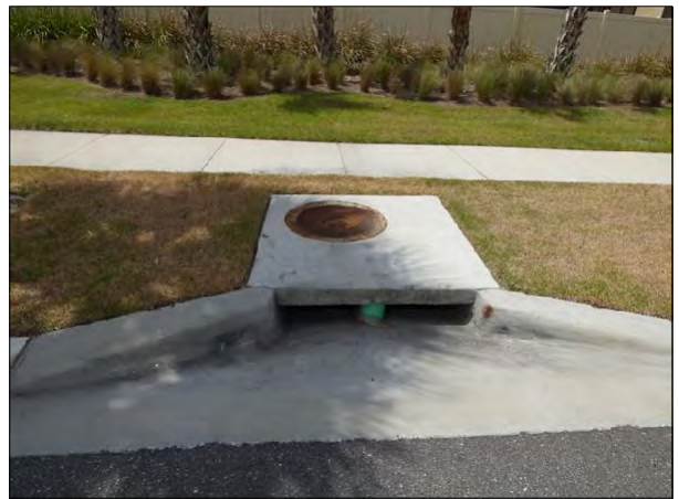
Stormwater Drainage Curb Inlet
