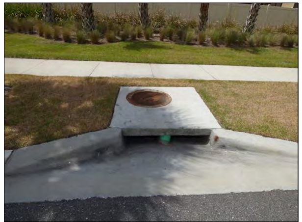
Stormwater Drainage Curb Inlet
