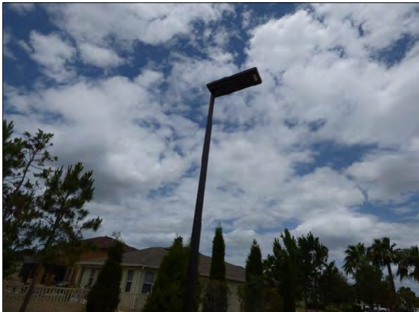
LED Playground Lighting
