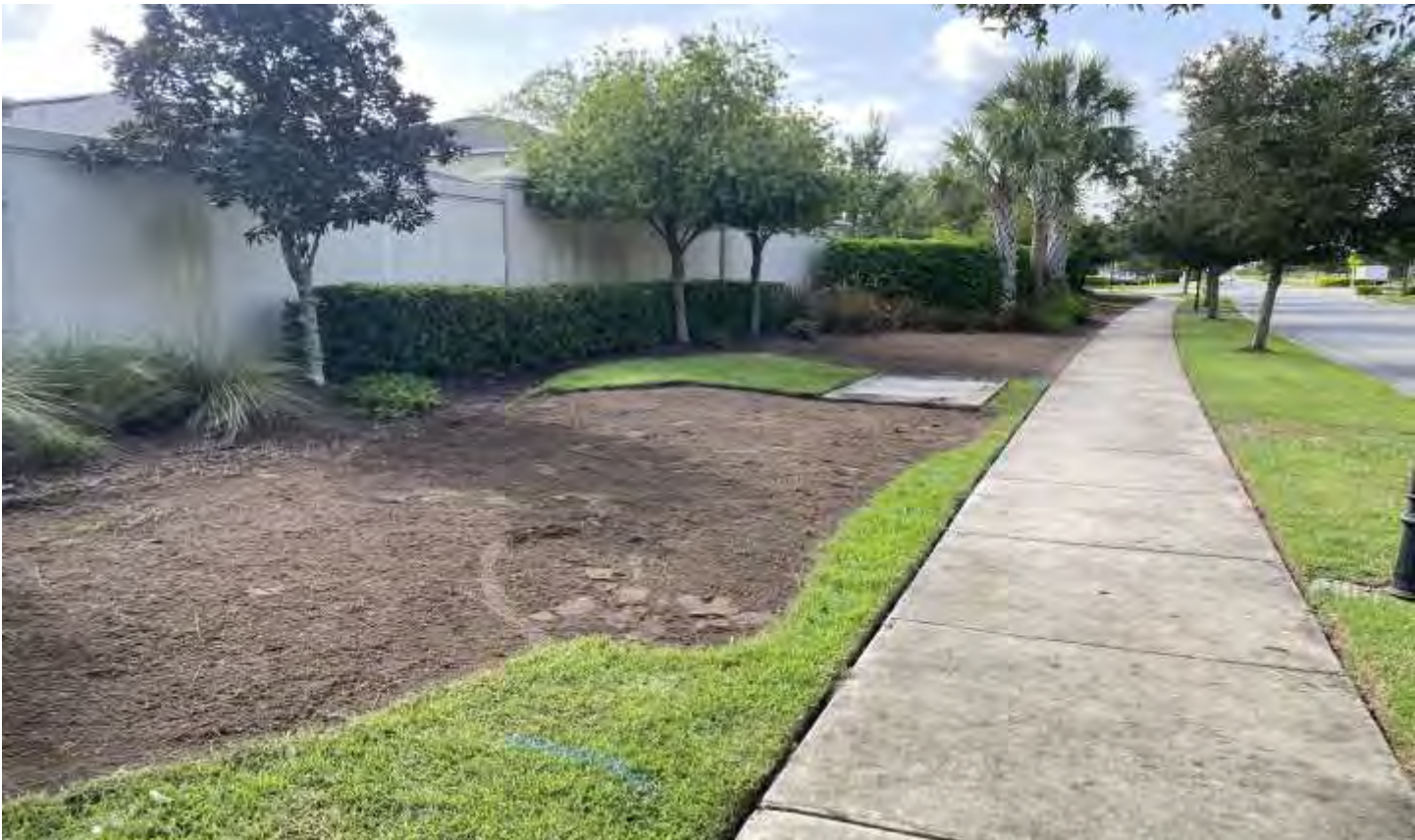
Brightview is prepping the east side of Summerfield Drive before the clubhouse for new sod.
